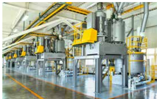
原料混合 Mixing equipment
